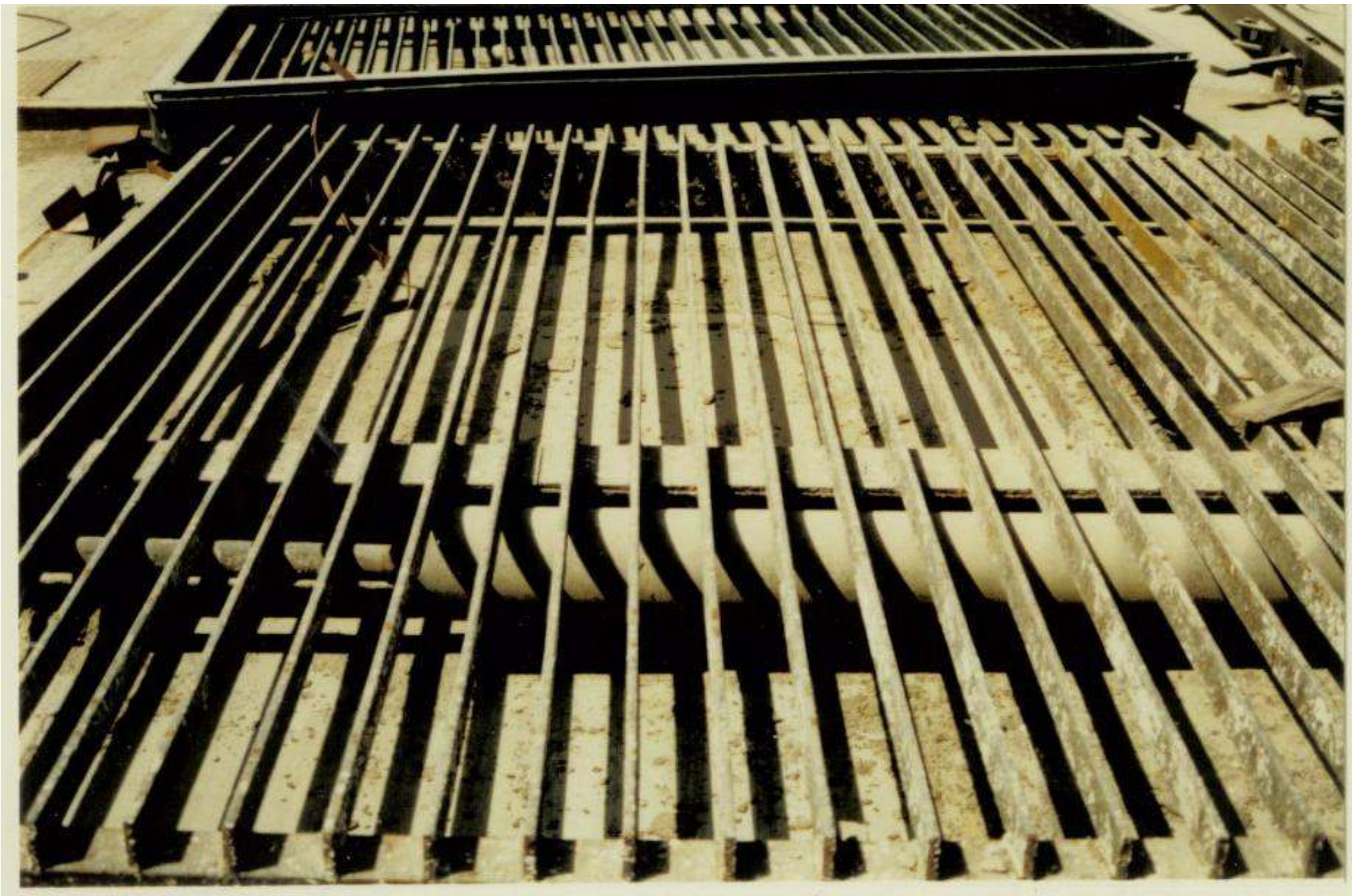
Screen bar 10cm wide at entrance of forebay
