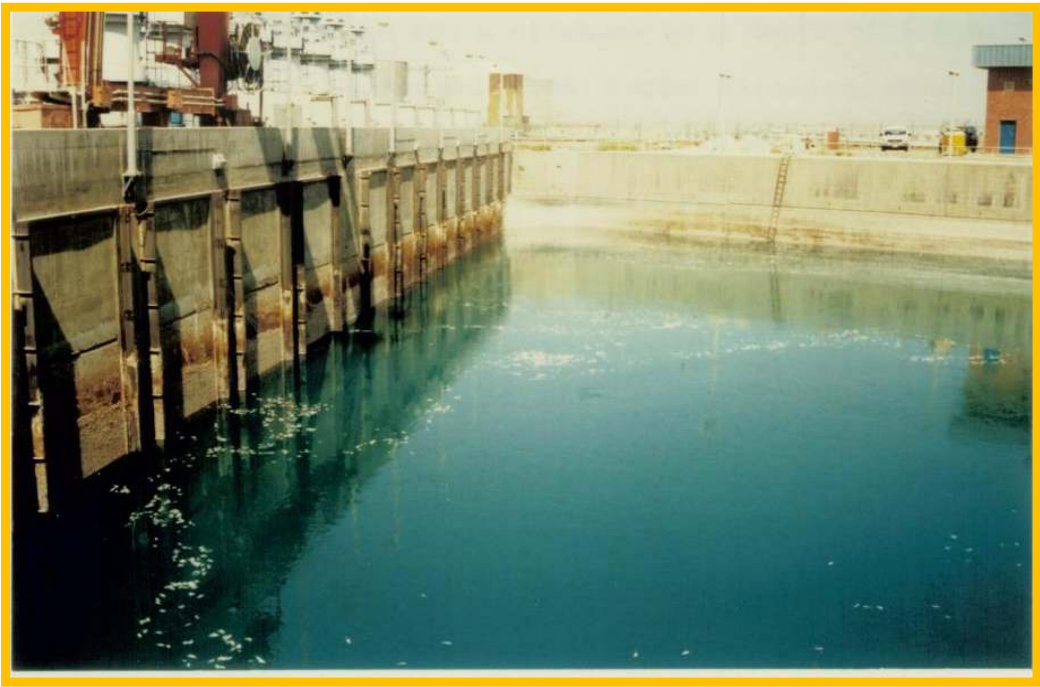
Forebay of a desalination plant intake
