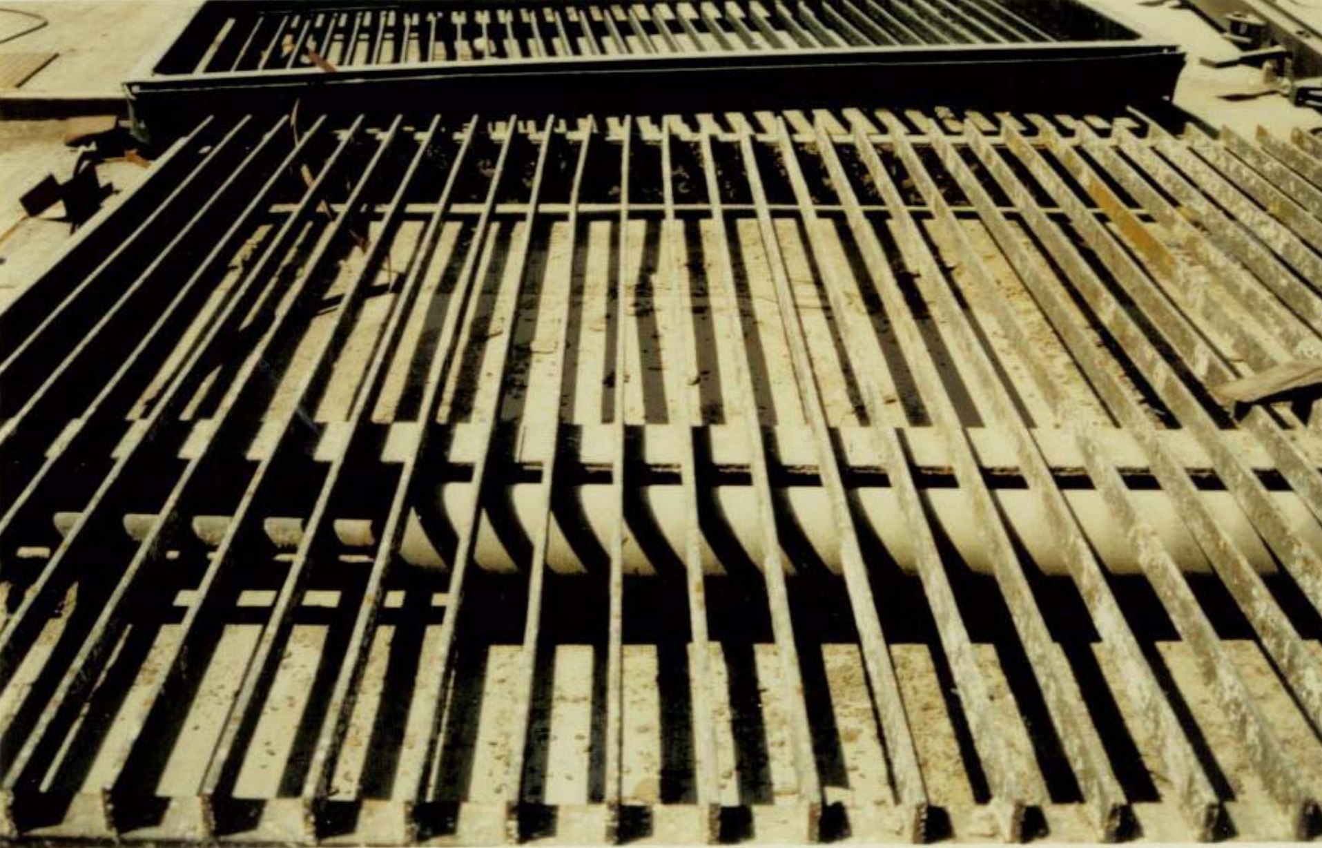
Screen bar 10cm wide at entrance of forebay
