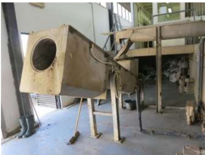
Figure 6 Screening s screw compactor discharging to a screw conveyor
