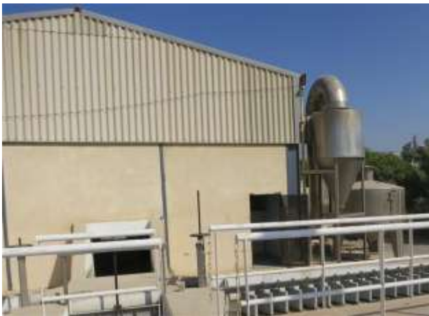
Figure 14 Screen house odour control (to right of photo)
