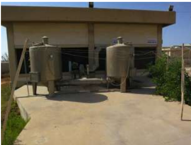
Figure 15 Outfall wet well Odour Control Unit (Activated Carbon)
