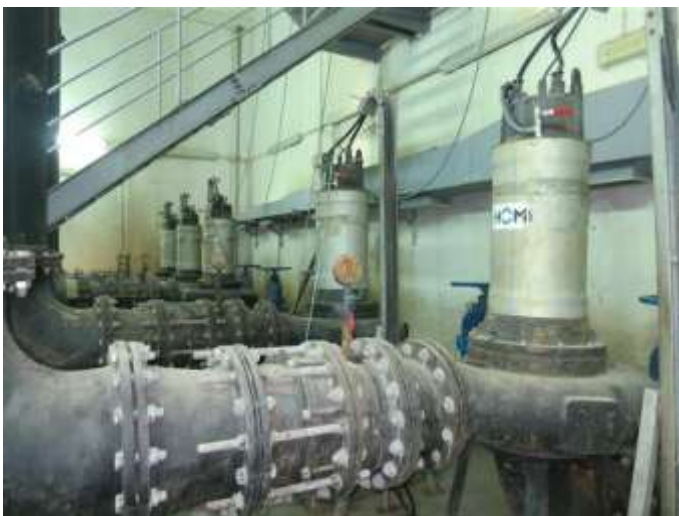
Figure 2 Saida Intake pumps station T1
