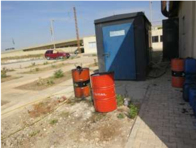
Figure 12 500 kVA generator in kiosk
