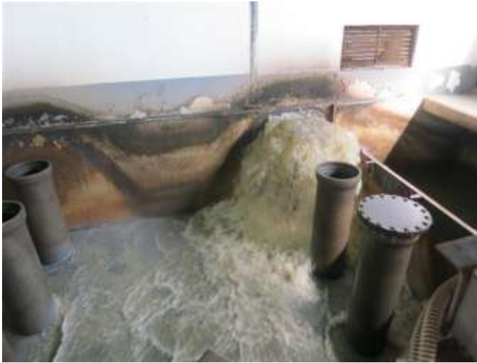
Figure 3 Intake pump discharge bell-mouths
