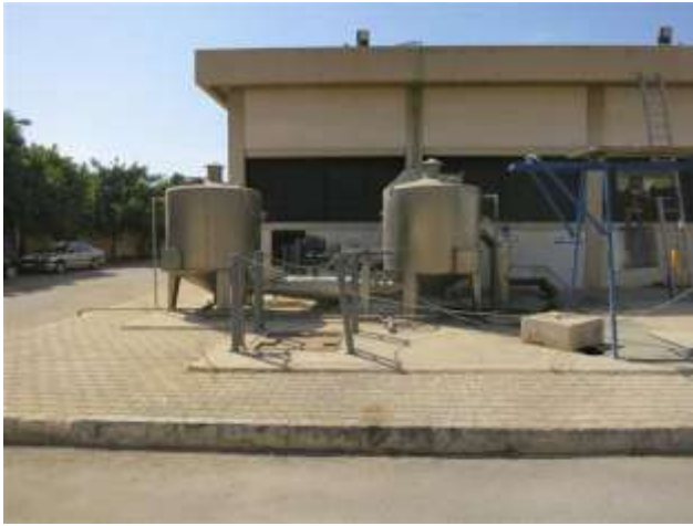
Figure 13 Intake well Odour Control Unit (Activated Carbon)
