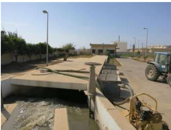
Figure 9 Outfall buffer tank
