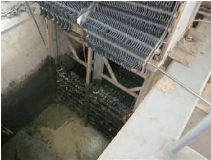
Figure 17 Fine Screen damaged by large objects
