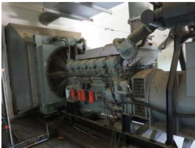
Figure 11 1280kV standby generator
